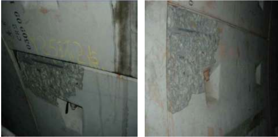
Figure 1: Damage to ordinary reinforced concrete shield segment
